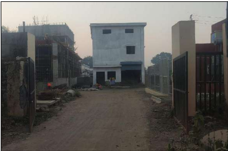
Figure 9 – Panchvati Water Treatment Plant
